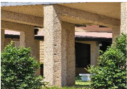
Picture: Courtyard pillar damage
