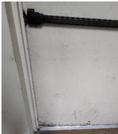
Picture: Damaged kitchen door
